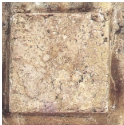
Oberfläche nach AC 4 Ag/SnO 2 SPW Surface after AC 4 Ag/SnO 2 SPW Surface après AC 4 Ag/SnO 2 SPW
